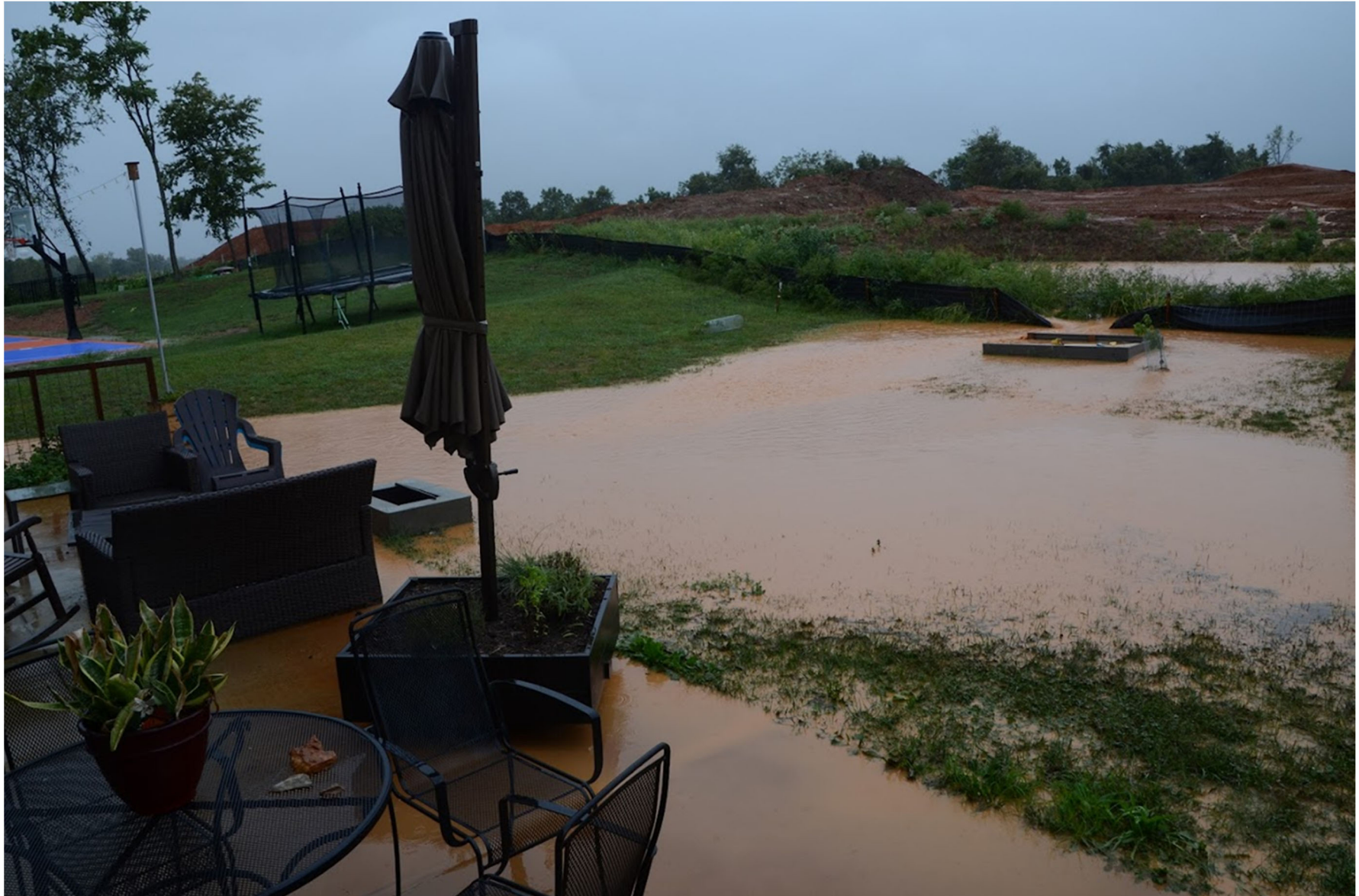
Run off near a construction site during a heavy rainstorm. Photo by Jon Burge. Used with permission.
